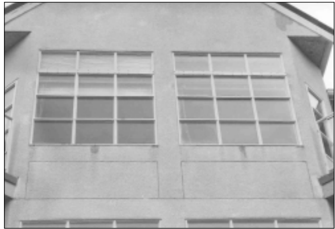
Figure 2. Example of localized wetting as a consequence of ineffective window-seal detail
